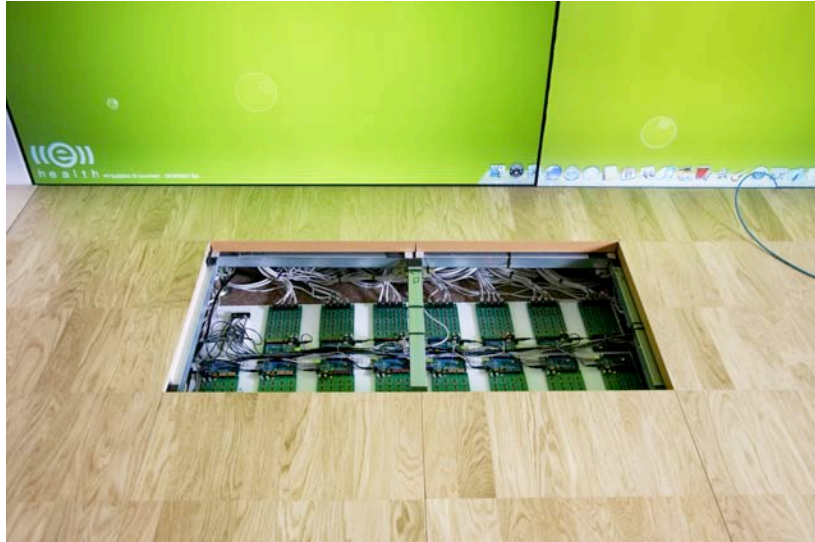
Image 2: operation amplifier and microcontroller boards under the metal support structure for the sensors and the floor tiles
